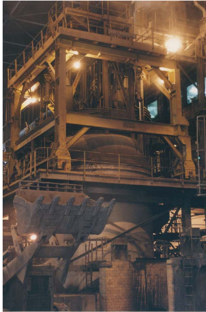
Vacuum tank, cover and cover car that transports the multi-ton cover. The cover is the portion of the equipment that contains all control devices and power connections required to produce stainless steel.
