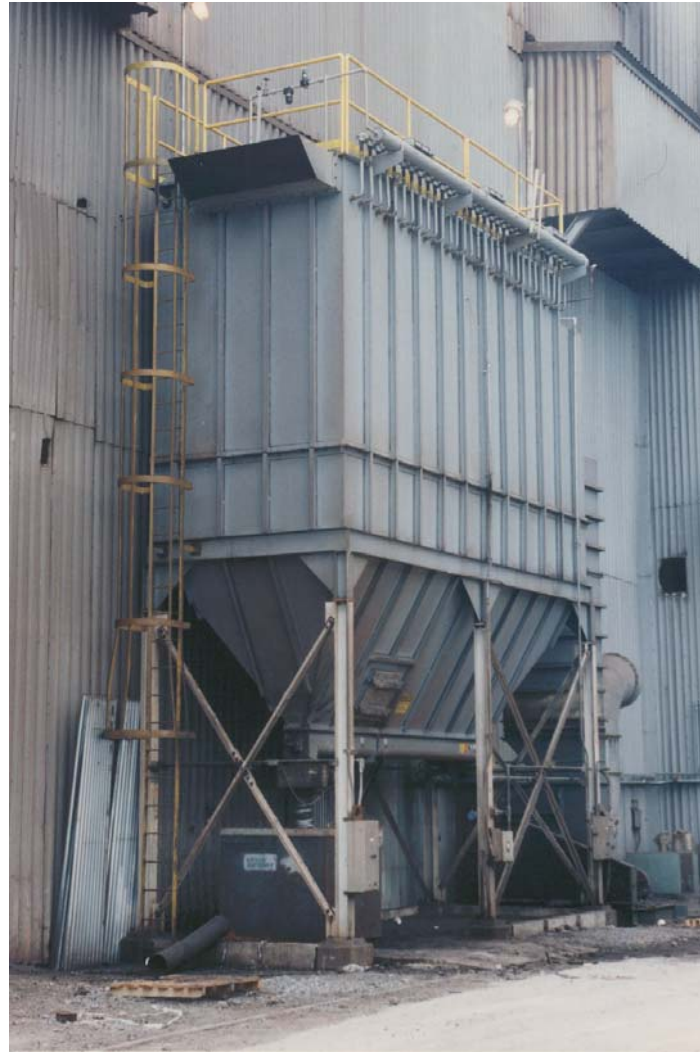
Bag house dust collector system that contains solid particulates removed from steel making process.
